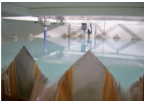
Onthardingsinstallatie in Kooigem
