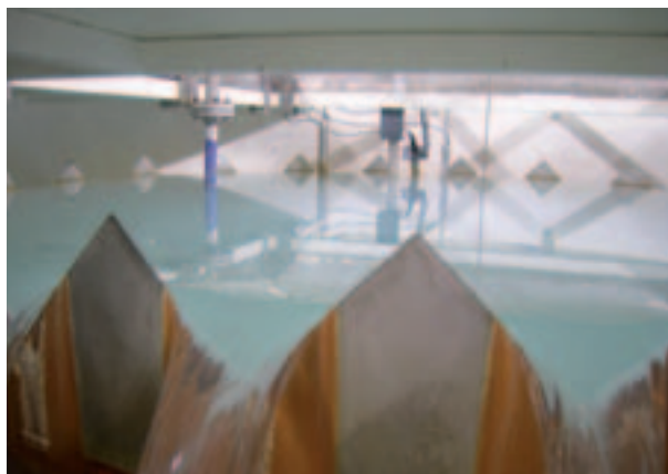
Onthardingsinstallatie in Kooigem
